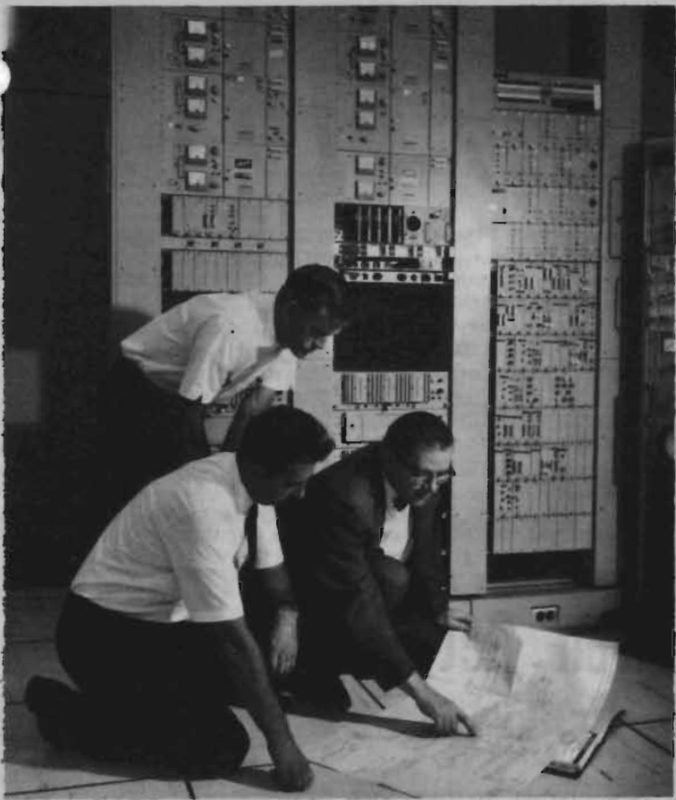
CHECK THIS - The Lenkurt 76C Microwave Radio installation at the Range Control Center is shown in the background as Bob Canavero, Lenkurt installation supervisor, left kneeling, and Chuck Parker, WSMR program manager for Lenkurt, examine over-all system plans. Ray McPherson, White Sands test technician, is pictured standing. (U.S. Army Photo by Robin Brown)
